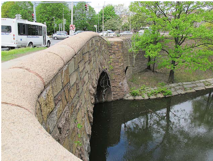
■ Figure 61. Past and present encountering, modern-day traffic traversing a historic bridge. Photo by Jeb Sharp 2015.
